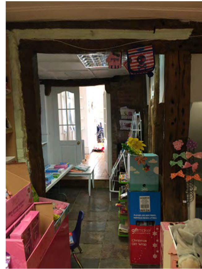
C) Original framing exposed to interior of toyshop, to be retained insitu.
