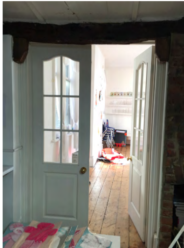
J) Infill location C. Partitions to sit within existing historic timber which will remain exposed to toyshop. Plasterboard infill will be scribed around historic timber details.
