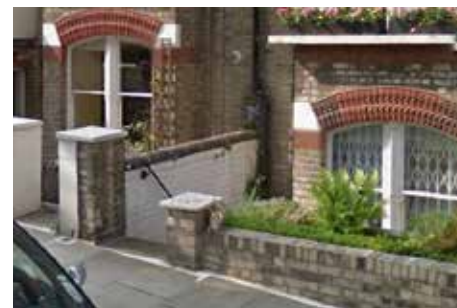
Existing access demonstrates markings that indicate the previous presence of a gate
