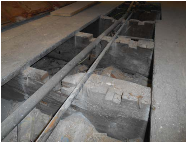
Photo 3: Notches to third floor rear room joists.
