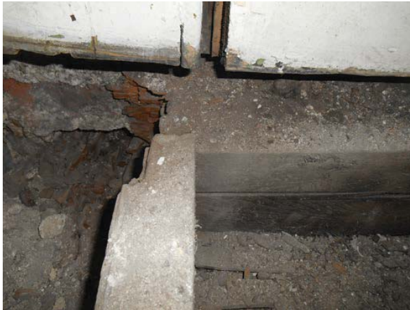
Photo 2: Rot to first floor beam end (beam A).
