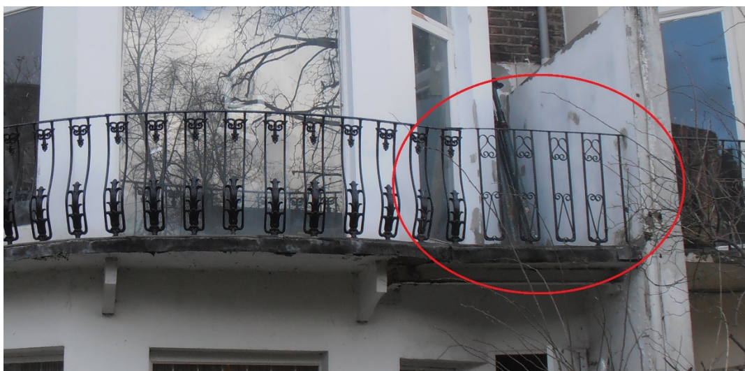
Balcony’s railing has different pattern on the side where the staircase was present (marked in red)
