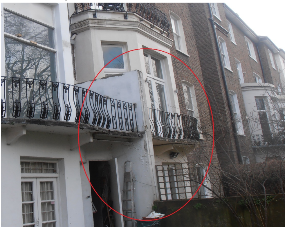
Boundary wall missing section (marked in red)
