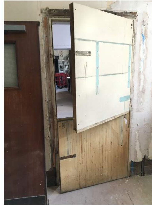
EXISTING STABLE DOOR - G.15 SIDE CAREFULLY REMOVE EXISTING DOOR FRAME COMPLETE AND CART AWAY
