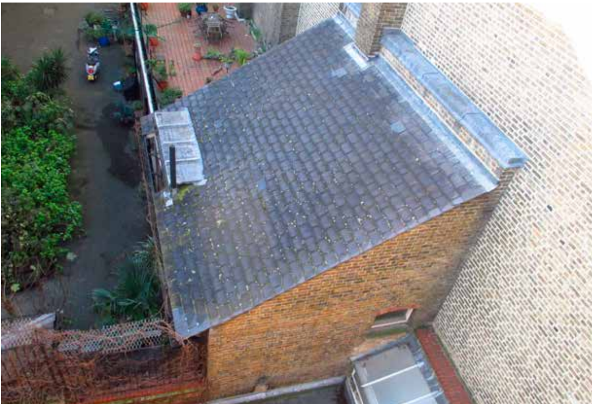
Fig. 3.4: Aerial view of slate mono pitch roof to 'house'. It is proposed that the slate is salvaged and reused where possible in the development
