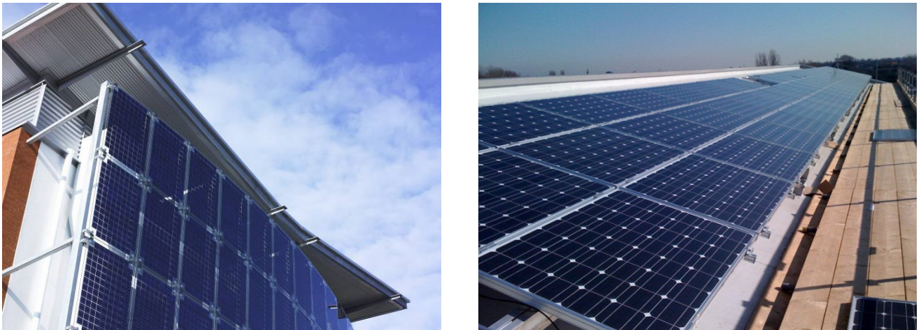
Figure 3. CPW Photovoltaic Installations: Project Epic (BREEAM Excellent Office – above left) and Castle Wood (BREEAM Excellent School – above right)
