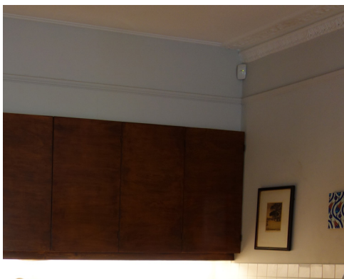
1. Loss of cornice to boxing in above
