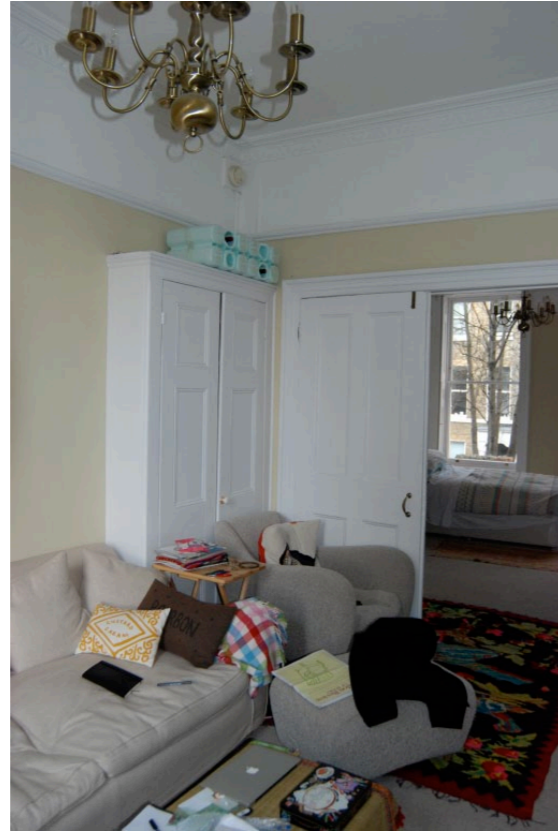
Double door opening to be partially infilled, nib to left to be removed to create new opening, and closet concealing doorway to be removed
