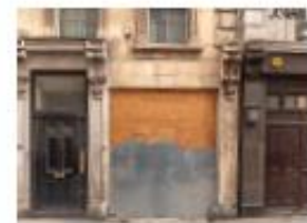
Inherited site in poor condition
