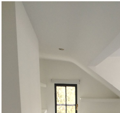
No coving at second floor.
