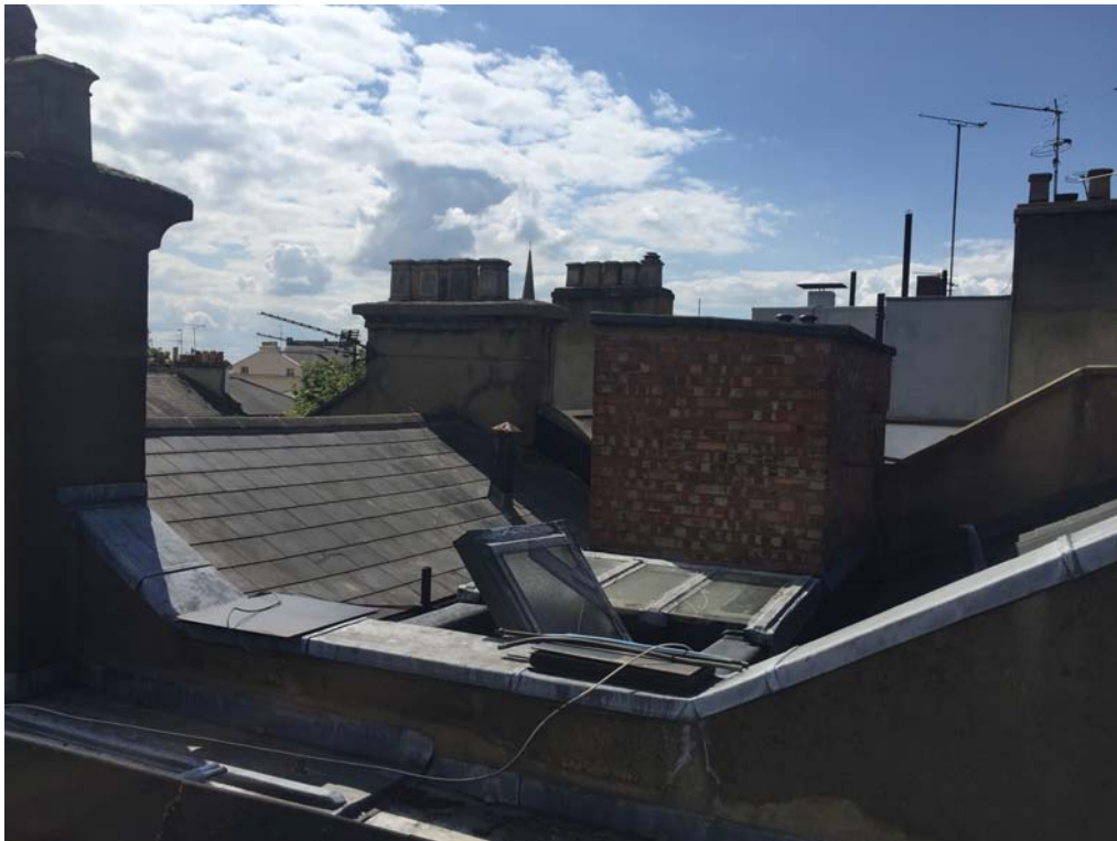
Photo 1 – existing roof, proposed extension would be between the brick water tank and the ridge line on the left of the photo.
