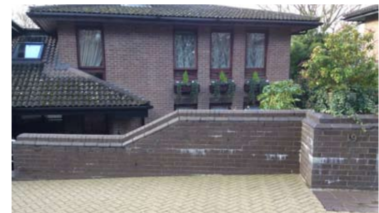
Image of sloping wall at the adjacent property (19 Highfields Grove)
