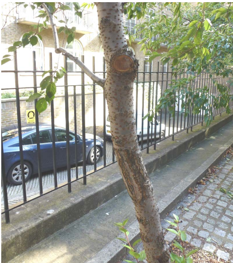
Image 07 Damage to T3 trunk and branch removal. Tree is leaning North and showing signs of stress due to epicormic growth at base of tree.
