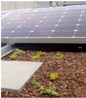
Green roof treatment with PV panels
