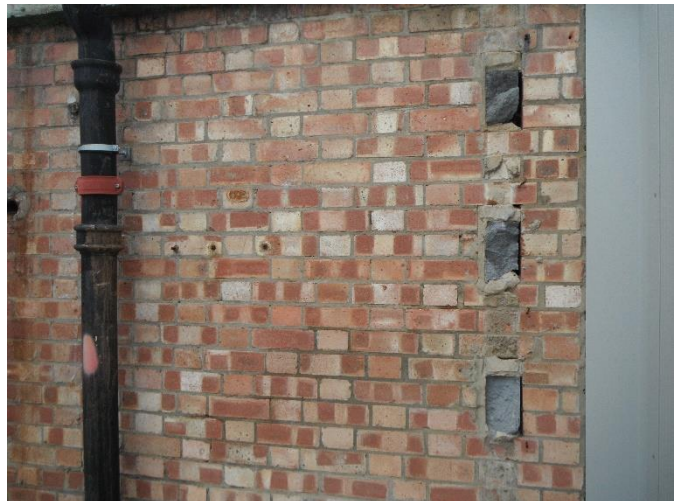
Photograph 3 Gaps in the brickwork of Building 1.
