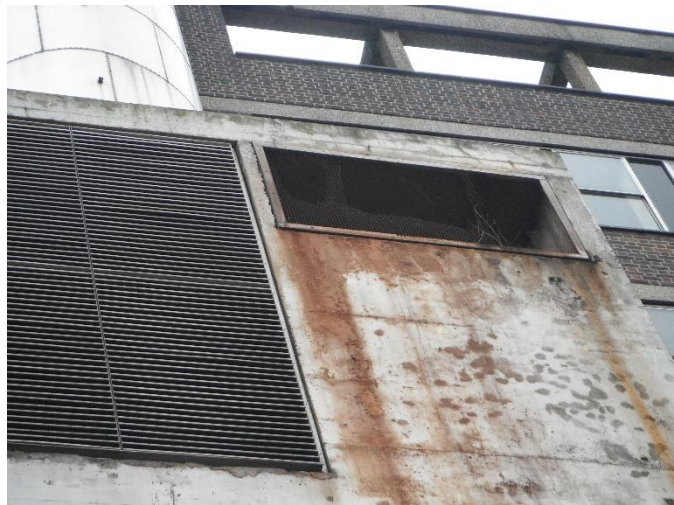
Photograph 2 Mesh coming away from an opening on the chimney tower of Building 1, providing opportunities for nesting birds.
