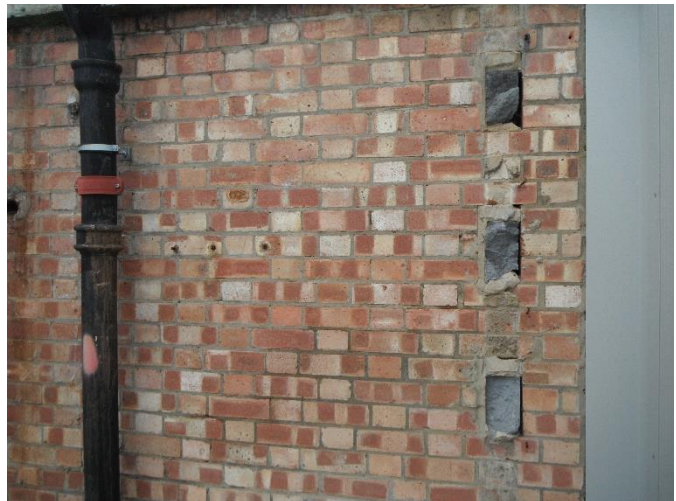
Photograph 3 Gaps in the brickwork of Building 1.
