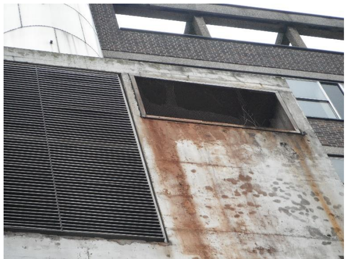
Photograph 2 Mesh coming away from an opening on the chimney tower of Building 1, providing opportunities for nesting birds.
