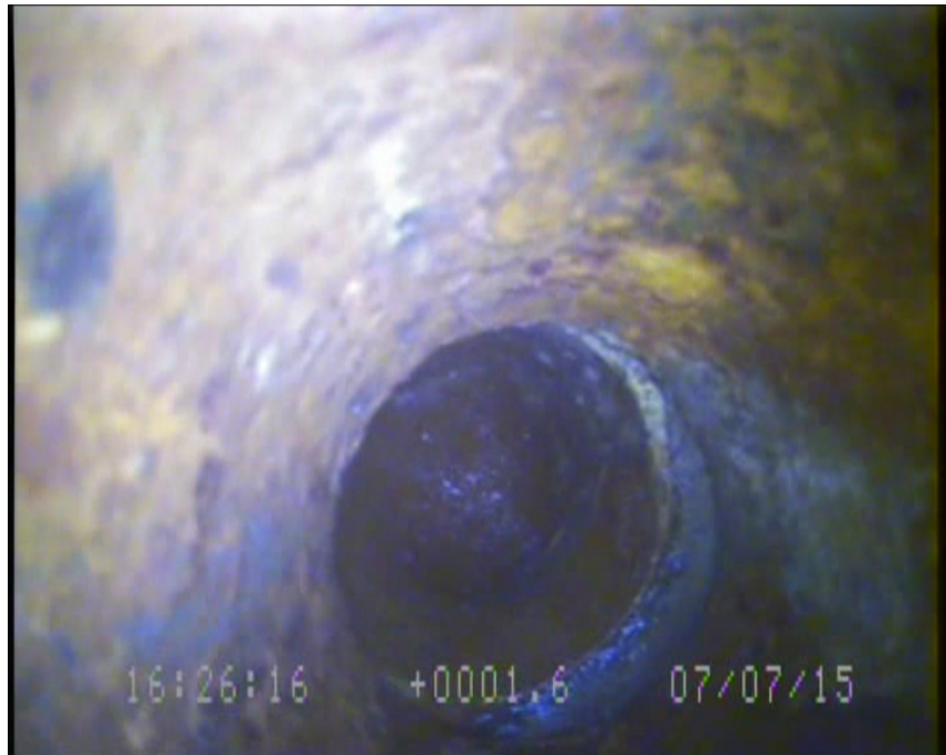
Photo: 1_1_6_A.jpg 1.6m, Open joint, 50mm of diameter
