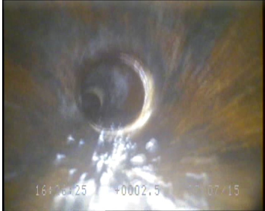
Photo: 1_1_9_A.jpg 2.6m, Joint displaced, medium
