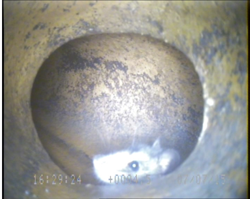
Photo: 1_1_14_A.jpg 4.6m, Vermin, rats observed in connection
