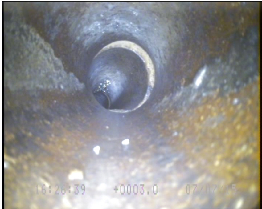
Photo: 1_1_11_A.jpg 3.2m, Joint displaced, medium
