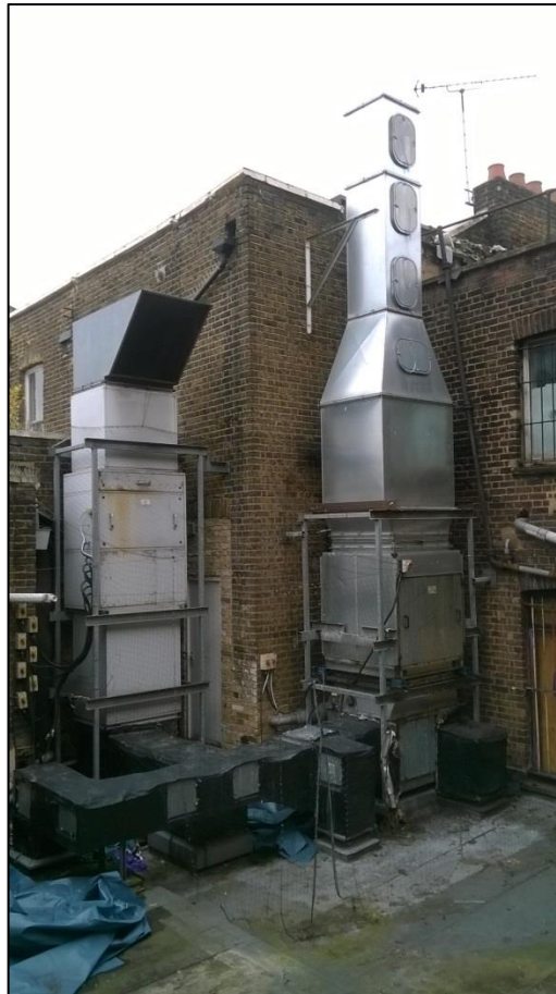
Figure 4.1: Kitchen Extraction Unit
