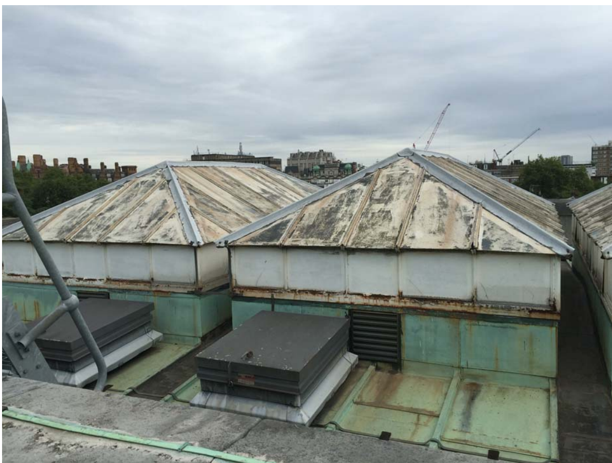
POOR SKYLIGHT CONDITION
