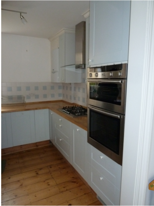
Kitchen with boiler in the corner.
