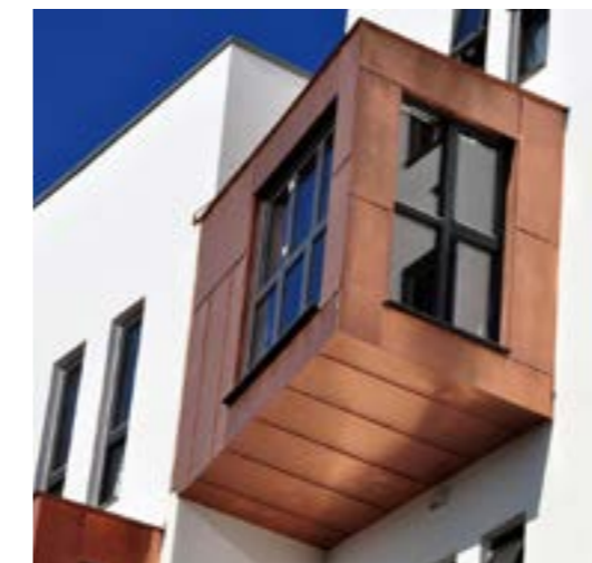
Example of relationship of copper to render cladding as proposed on rear elevation of development.
