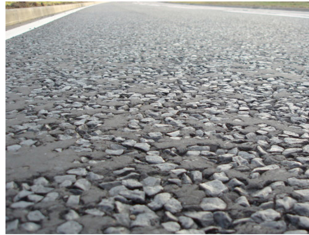
Typical Image Of Hot Rolled Asphalt With Exposed Aggregate (P8 & P8A) - Areas Of Tybalds Close To Be Constructed To Highways Adoptable Standard Exact Details To Be Confirmed With Local Highway Authority Scale: 1:20 at A1
