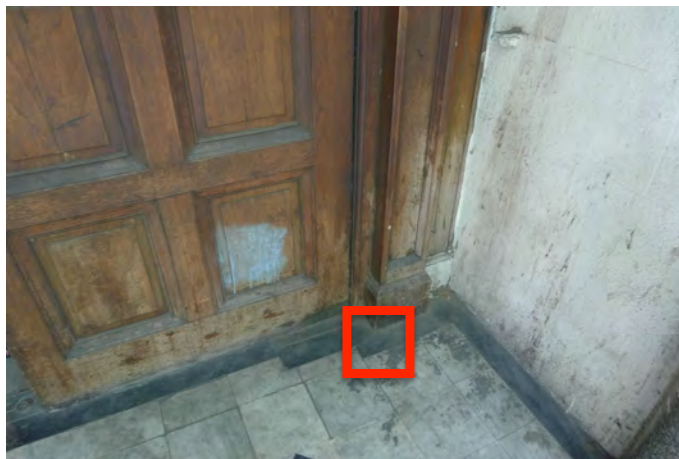
Fig 1: Southampton Row Entrance, floor detail indicating proposed location of recessed floor lights.
