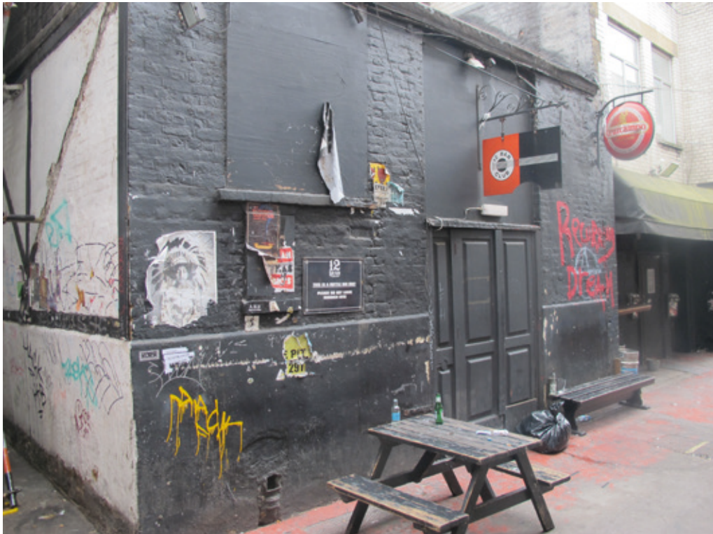
No. 22, the north façade to Denmark Place, showing blocked windows and modern applied timbering (left)
