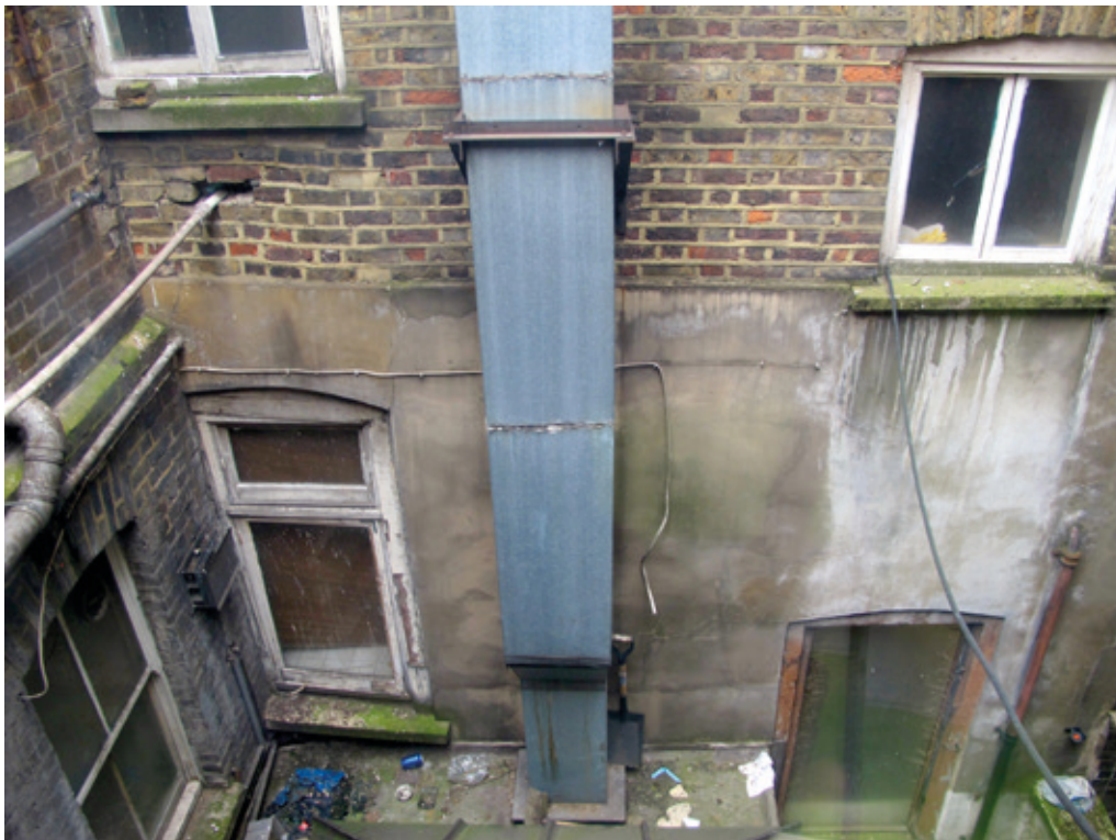
Rear of No. 26, showing the altered window (lower right)
