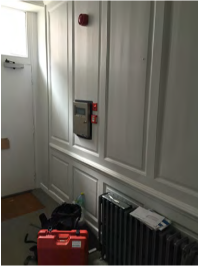
Fig. 25- Entrance Fire Panel
