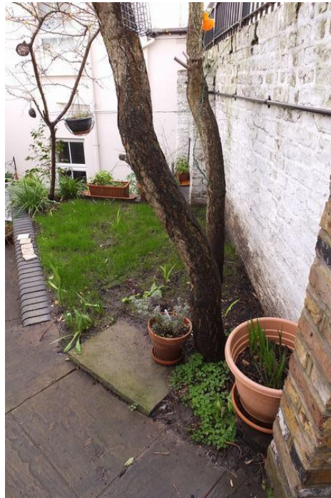
Image 3 Stems of T1 and T2 showing their proximity to the wall.
