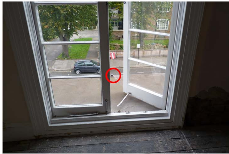
Photos taken on site at No. 47 UPR show evidence of a balustrade in place across the front of the roof of the bay window located at the front of the property
