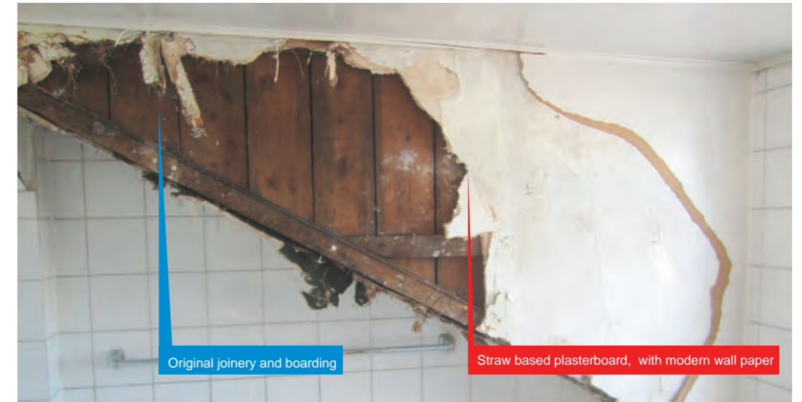
North side of attic space, view from bathroom, with damaged plasterboard removed to examine for water leaks from outside
