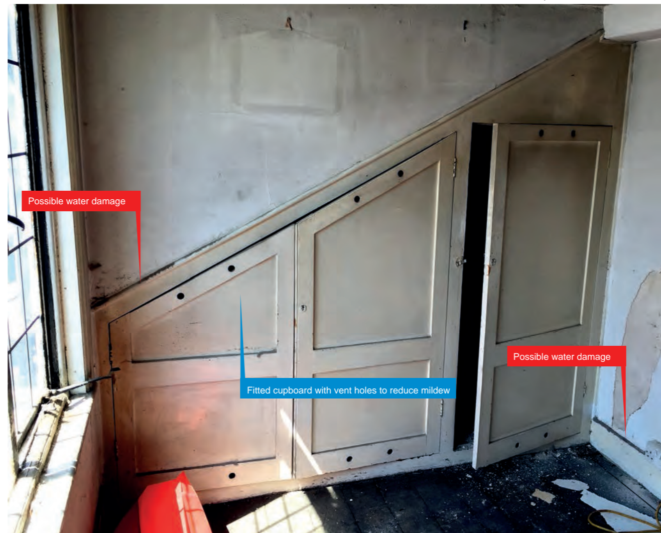
Living room, north wall, with fitted cupboard and showing possible signs of water ingress along top edge and damage to base of partition of the right, between common stair and living space.
