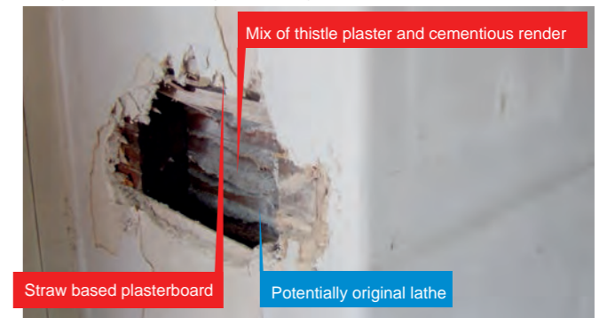
Living room, partition open to see composition and potential fire risk.
