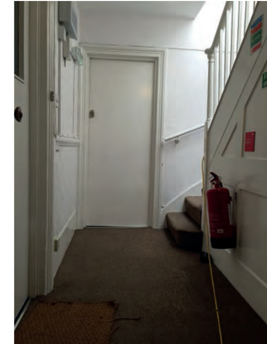
▲ Third floor landing : potential to create self contained demise, with new front door located at this level. Note door in picture is a permanently locked door to the flat on the third floor. It is not an emergency exit.
