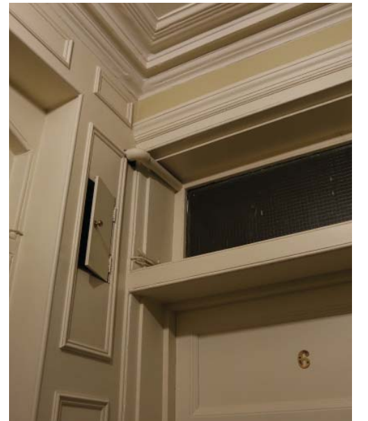
FLAT 4 ENTRANCE DOOR AND SERVICES
