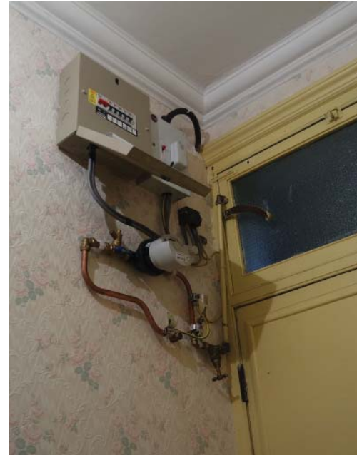
EXPOSED SERVICES FLAT 7
