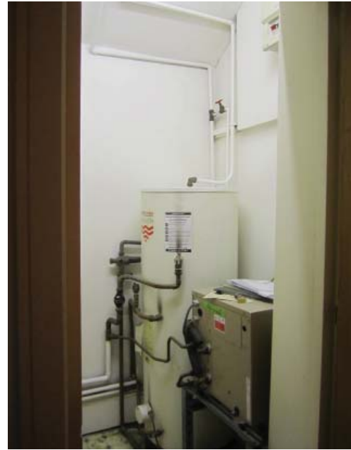
EXISTING PLANT IN STUDIO
