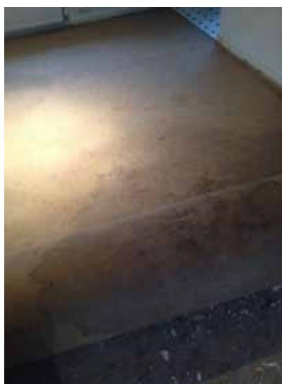
Fig 42. Existing water damage to third floor
