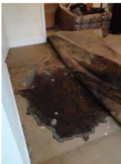
Fig 41. Existing water damage to second floor
