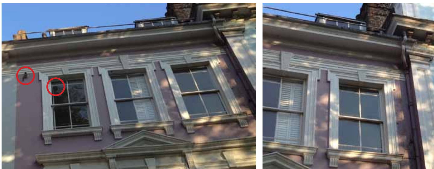
Fig 40. Existing water-damage to front elevation. Extract and flue to second storey to be removed.
