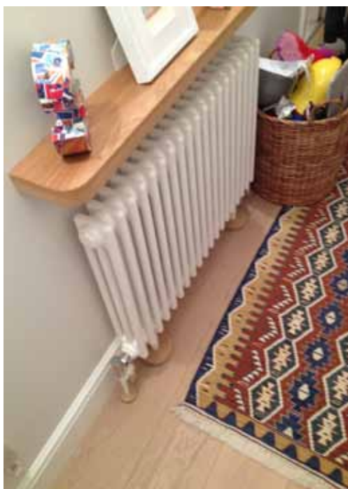
Fig 38. Existing column radiators to maisonette
