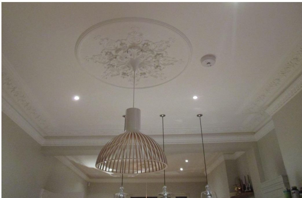
Figure 3.27 – Modern cornicing has replicated the historic design and reinstated legibility of the historic two-room plan form
