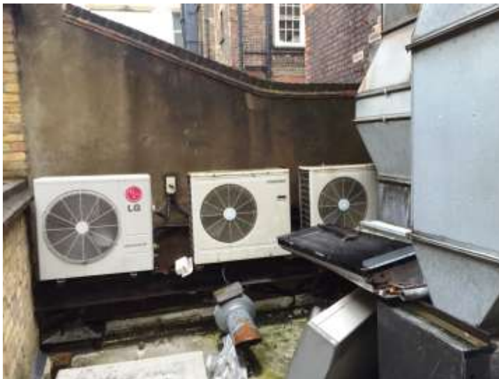
existing flat roof with 3 AC condensers
