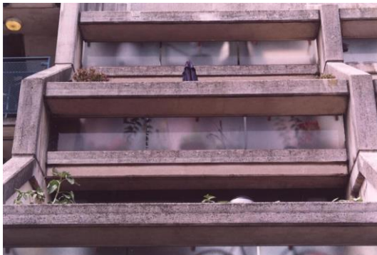
Proposed: Staining removed
