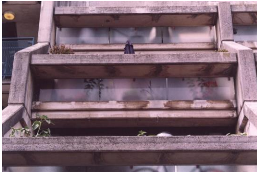
Existing: Staining to planters
