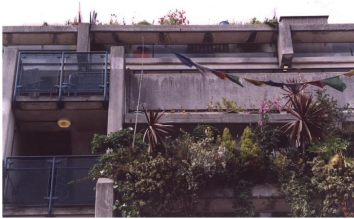
Existing - Streaking under balconies
