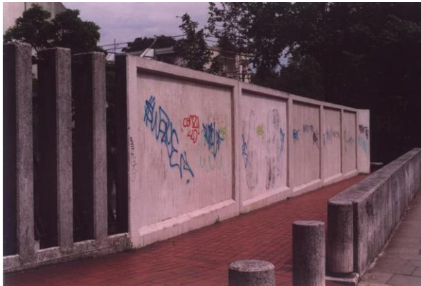
Existing: Graffiti on recently cleaned concrete.
