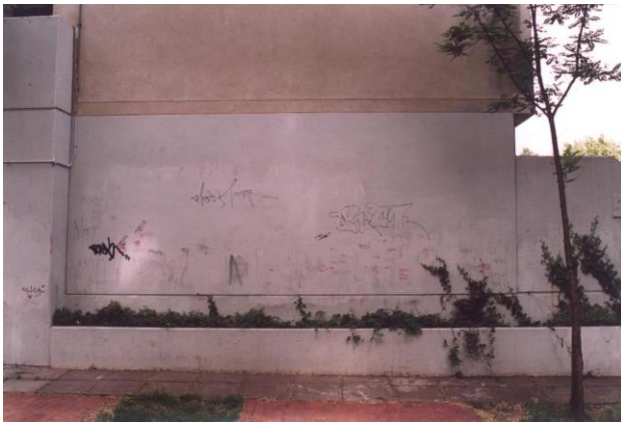
Bottom panel of render painted in with adjacent concrete – Architectural clarity lost.
