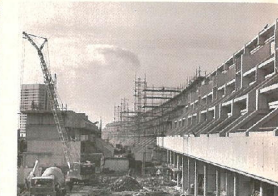
Left: the controversial surface-mounted lighting system that replaces conduit originally concealed within the concrete. Centre: one of the patched areas of concrete. Camden says this is still to receive a top dressing coat. Below left: detail of water penetration at a roof expansion joint, as drawn by Forbes Bramble Associates in the study of the estate before the present repairs were undertaken. Above: the estate in 1976. A detailed account of construction methods appeared in AJ 8.9.76
