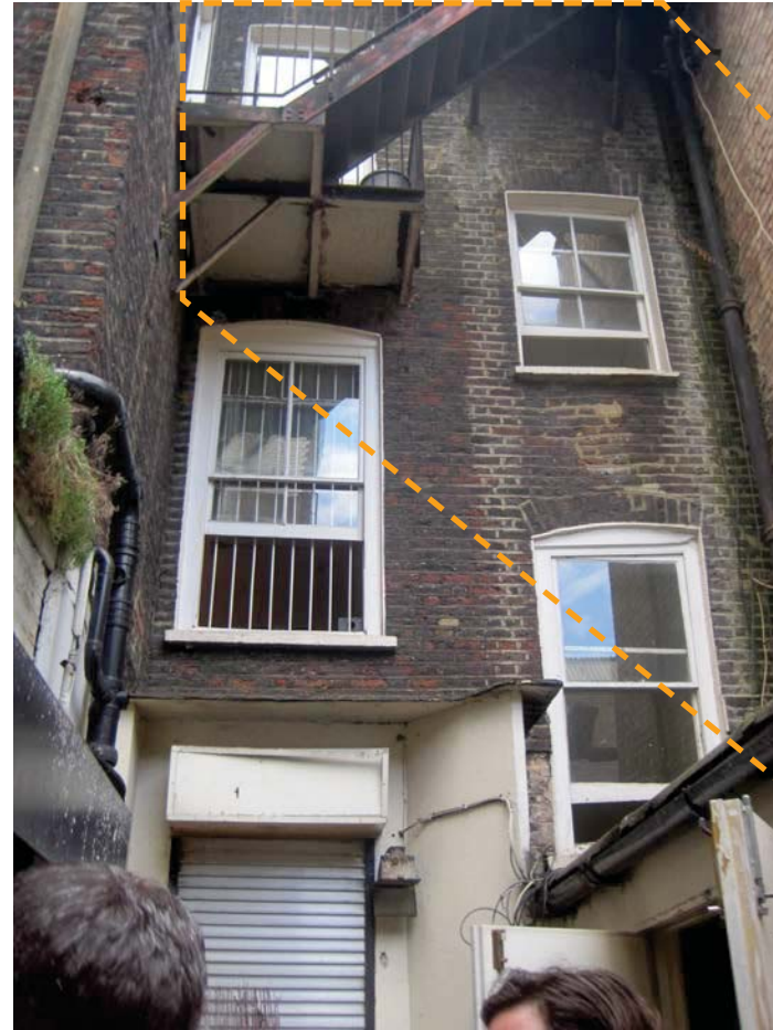
Existing rear elevation of townhouse with loss of legibility due to later accretions
