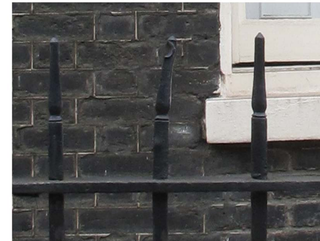
IMAGE OF DAMAGED FINIAL TO BE REPLACED TO MATCH ADJACENT
