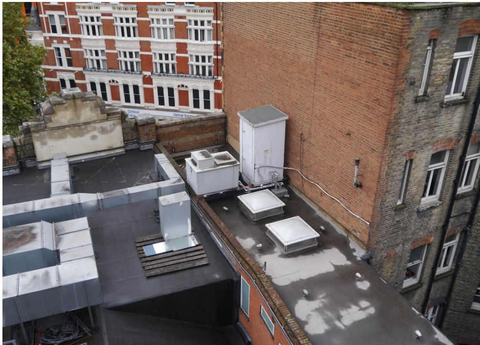
Above - Existing roof plant above modern extension which forms the Front of House Female WC. Plant and 2no. roof lights to be removed.
