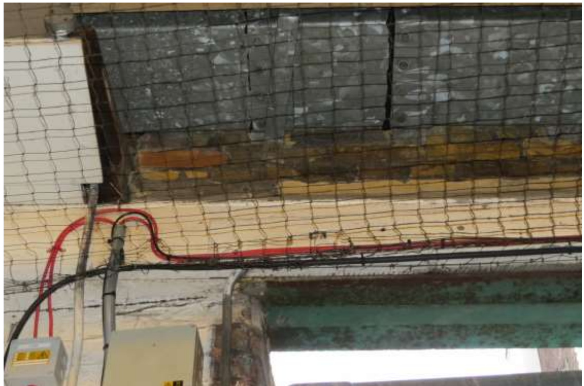
Photograph 2: Bird netting covering the full extent of the roof likely impedes access to any potential roost features.
