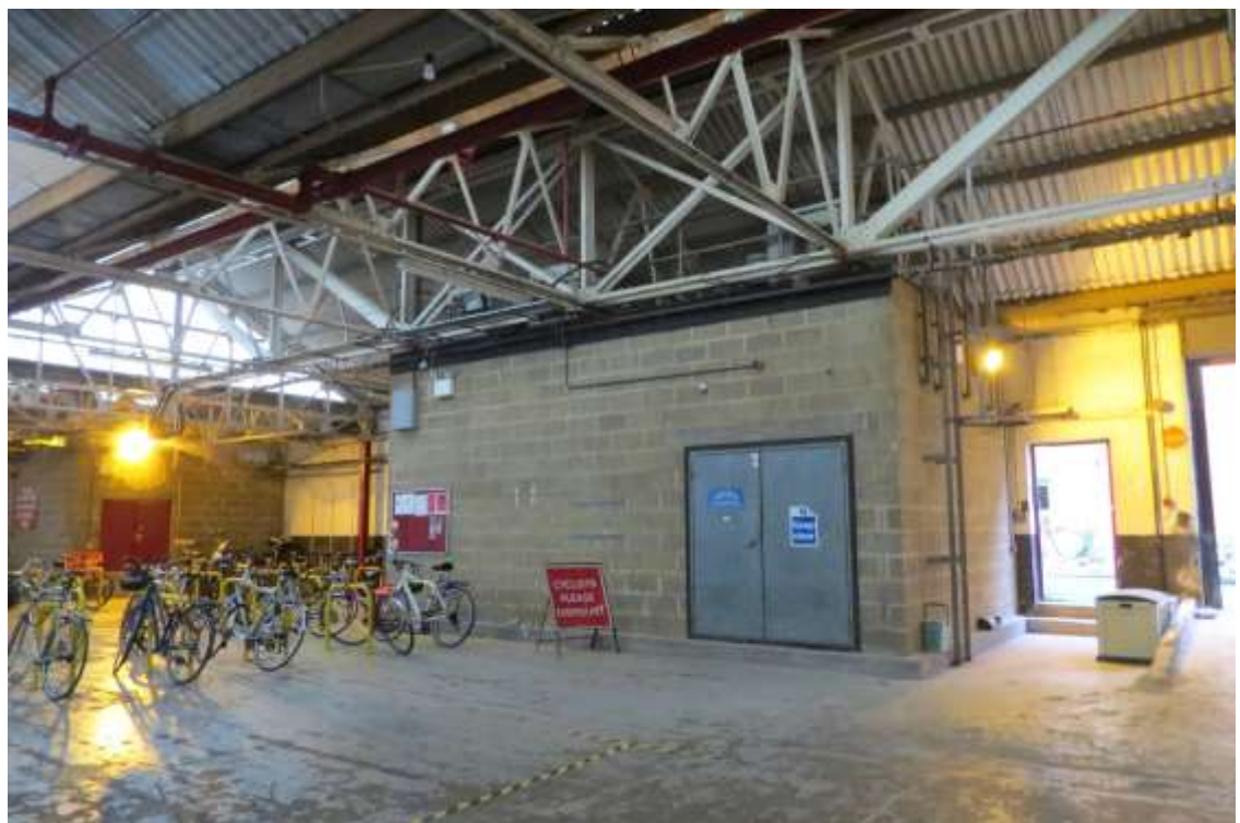
Photograph 4 (TN2): Electricity substations were well sealed and offered no opportunities for bats to enter into these structures
