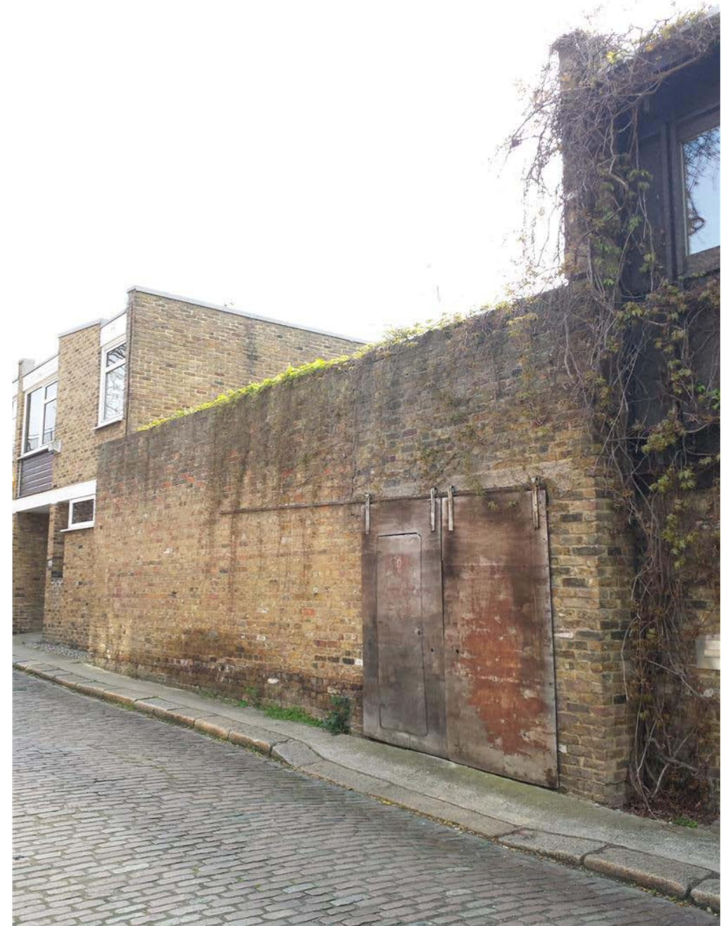
② View of the existing brick wall looking east from Camden Mews
