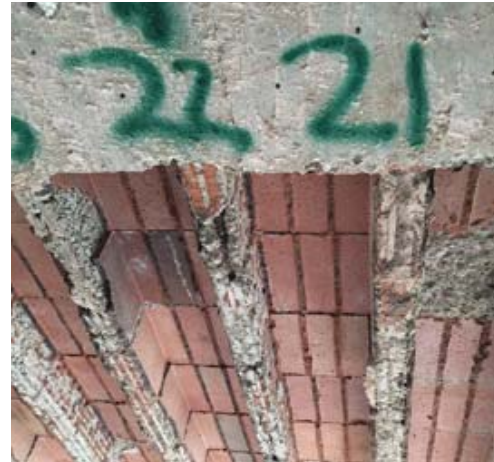
Varying cover to reinforcement bars - durability repair required
