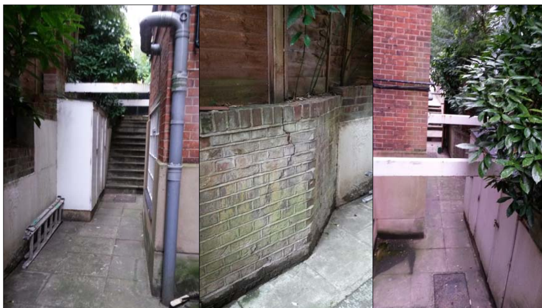
Left: Access via side of house, Middle: Cracking to adjacent retaining wall, Right: Struts between house and retaining wall
