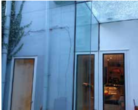
IMAGE 2.9. REAR DOORS + CONSERVATORY BROKEN GLAZED ROOF
