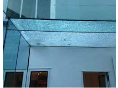
IMAGE 2.10. CONSERVATORY GLAZED ROOF BROKEN PANEL
