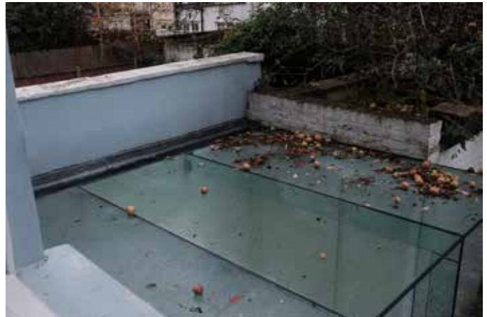
IMAGE 2.20. VIEW OF GLASS EXTENSION JUNCTION WITH BOUNDARY WALL AND BRICK SHED FROM GROUND FLOOR REAR WINDOW
