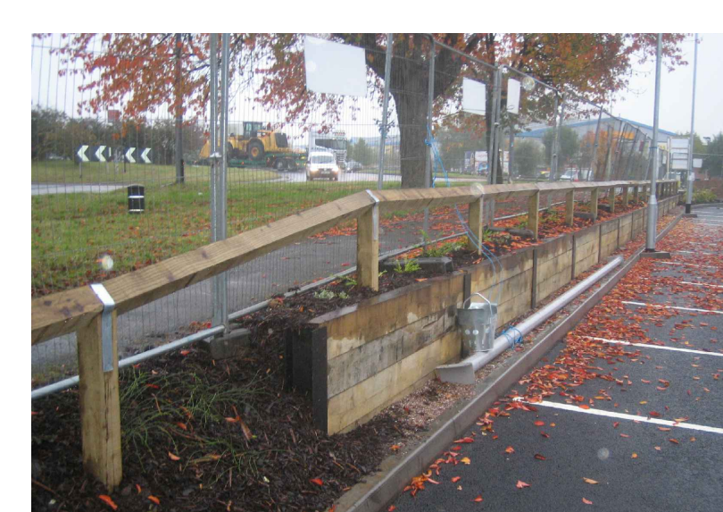
3. 1m high max timber sleeper wall with 3m high security mesh fence type 358 situated at highest profile.
