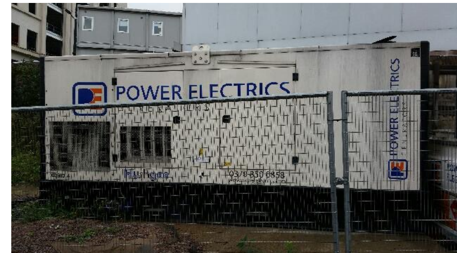
Super silent generator unit
