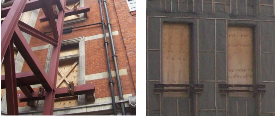
Figure 4 Typical connection detail via façade opening: External view (left). Internal view (right).
