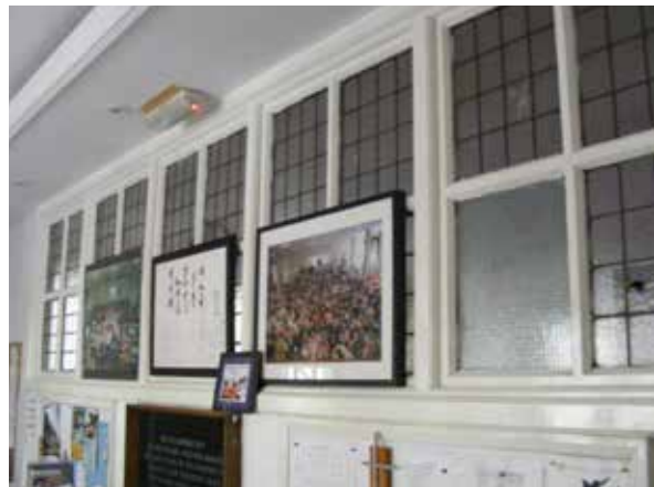
The leaded glazing between the lobby and the chapel is one of the very few remaining features - these are of late 19th century date.
