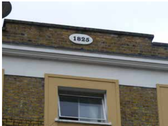
The 1825 datestone has been planted on an altered parapet which used to form part of the front pediment, removed when the roof was taken down to create the top floor flats.
