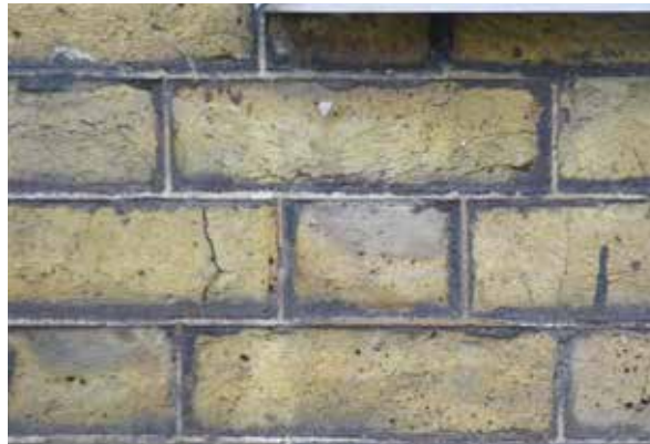
There are some sections of tuck pointing on the front elevation, where this has not been repointed or altered.
