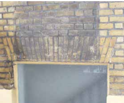
The gauged brick lintels on the remaining basement windows are indicative of the original build quality, although these remaining details are few.
