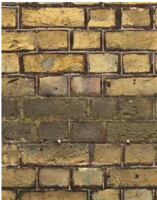
Original lime tuck-pointing has been replaced by large areas of cement-based repointing. The quality and consistency of the pointing overall is poor.
