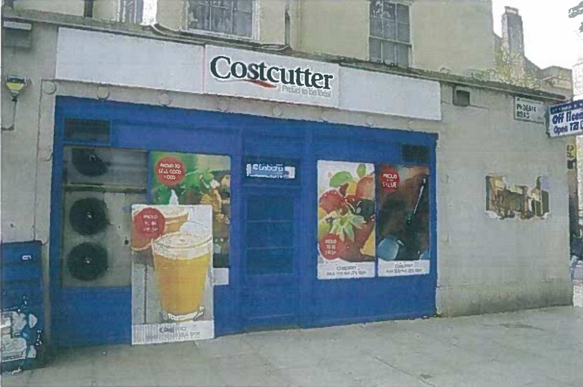
The Phoenix Road façade of 100 Chalton Street, showing the holes cut in the window for venting plant.
