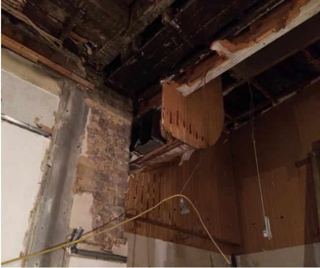
Remnants of previous flue
