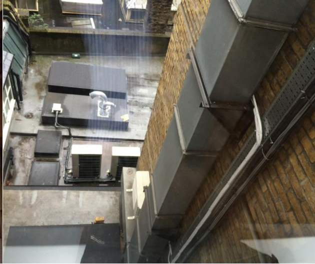
Plant machinery on ground floor roof
