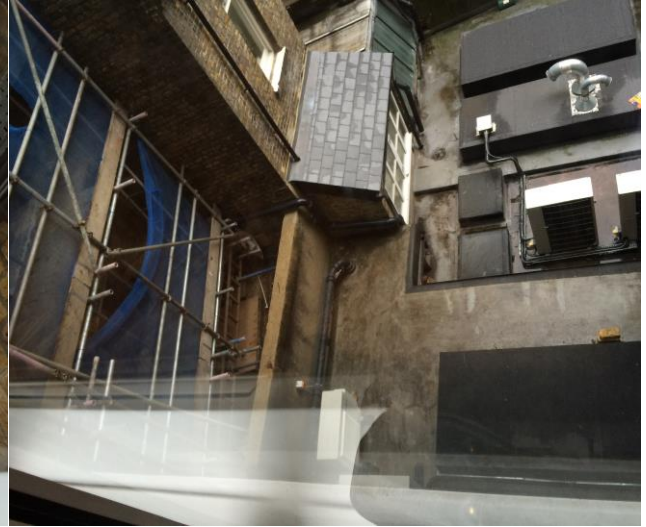
Plant machinery on ground floor roof
