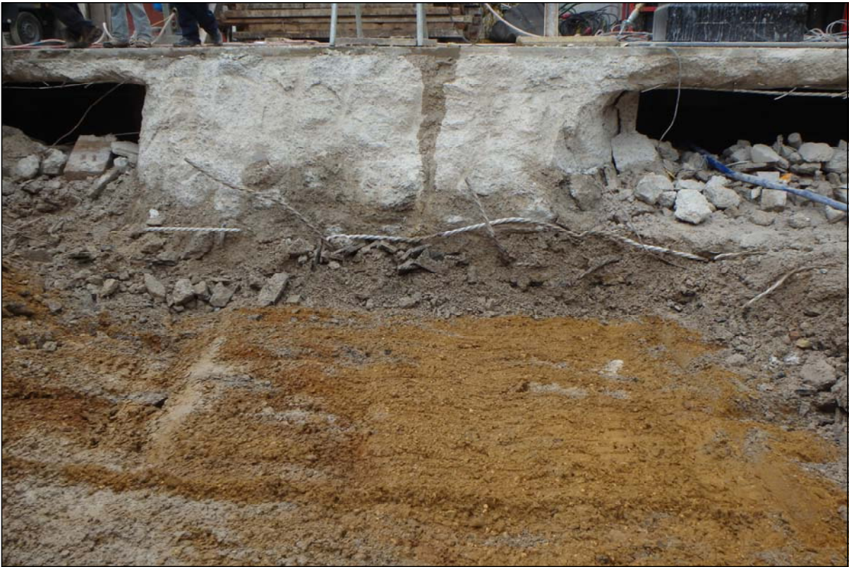
© Archaeology South-East 1 Bedford Avenue, London Fig.3 Project Ref: 6996 Aug 2015 'Time Out' building showing 2m thick concrete slab over natural sands and gravels, facing west Report Ref: 2015309 Drawn by: APL
